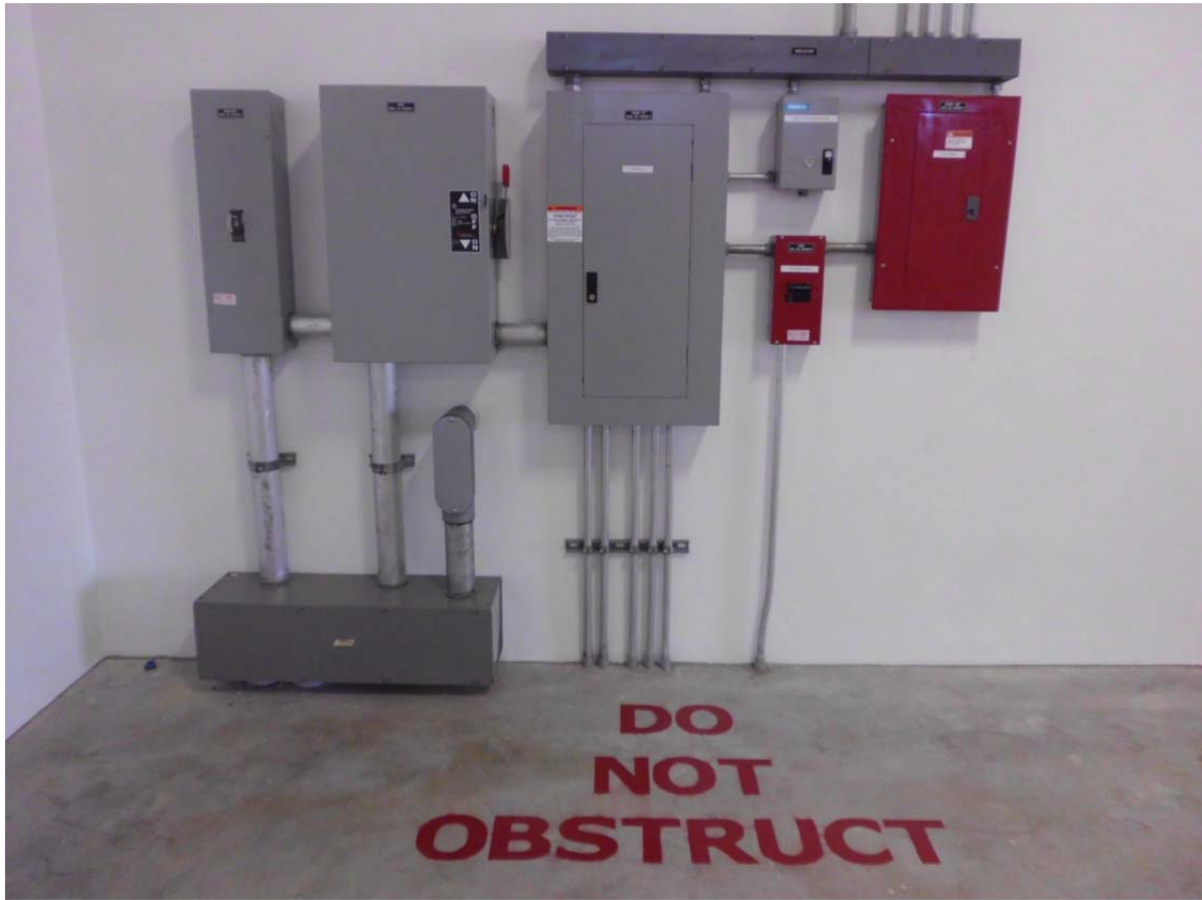
ELECTRICAL PANEL BOARDS
