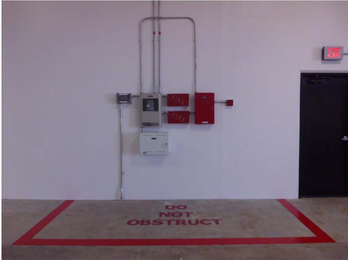
FIRE ALARM SYSTEM CONTROL PANEL & TRANSMITTER
